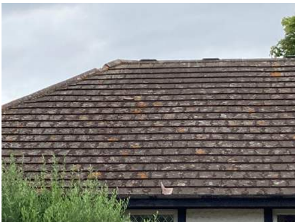
Missing ridge tile (southern aspect)
