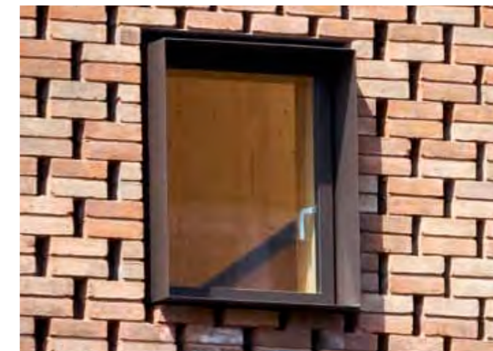
4. Protruding metal framed windows.
